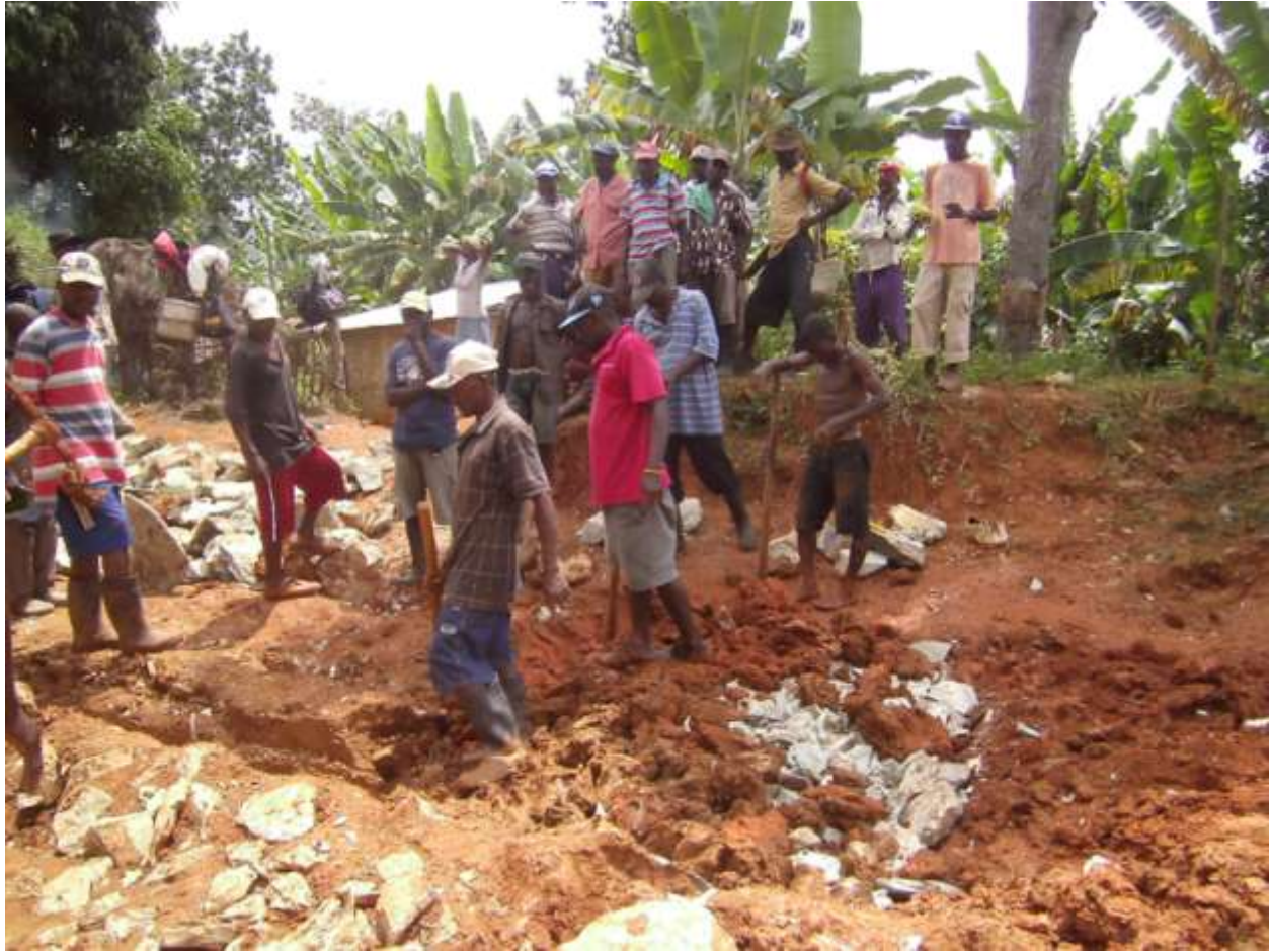
Work on the wroad in front of the gate of the church last Friday.
